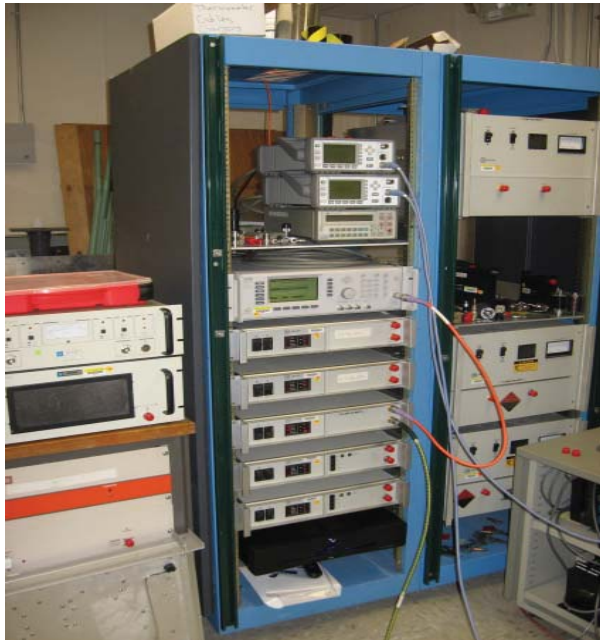
Figure 1. The instrumentation used to generate RF power. Two power meters (top) record the incident and reflected powers. Solid state (left), 20 W (center) and 200 W (right) TWT amplifiers are used below 1 GHz and 1 GHz to 18 GHz, respectively. A power regenerator (bottom) powers all the instruments.
